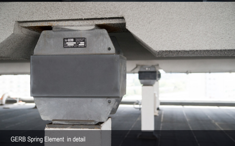
Spring supported helipad in Bydgoszcz
